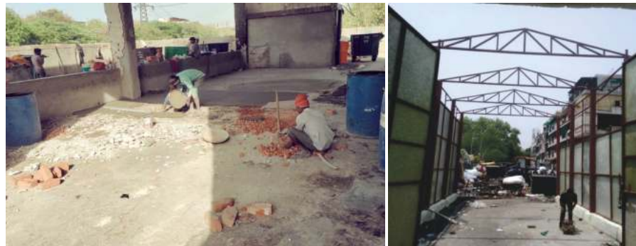
Work in Progress at Material Recovery Facilities in Patparganj and New Seemapuri, New Delhi
